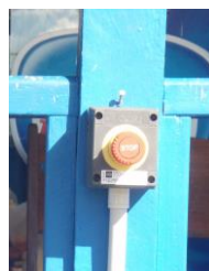
Figure 4: Emergency fuel pump stop button must be readily accessible.
