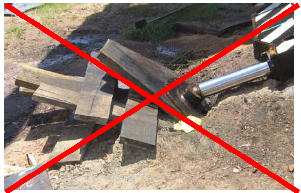
Photo 4: Example of poor ground & inadequate support
