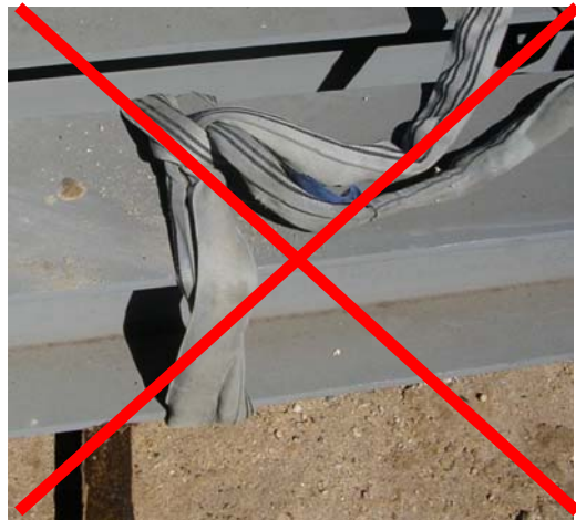
Photo 5: Synthetic slings without protection around beam – this is unacceptable
