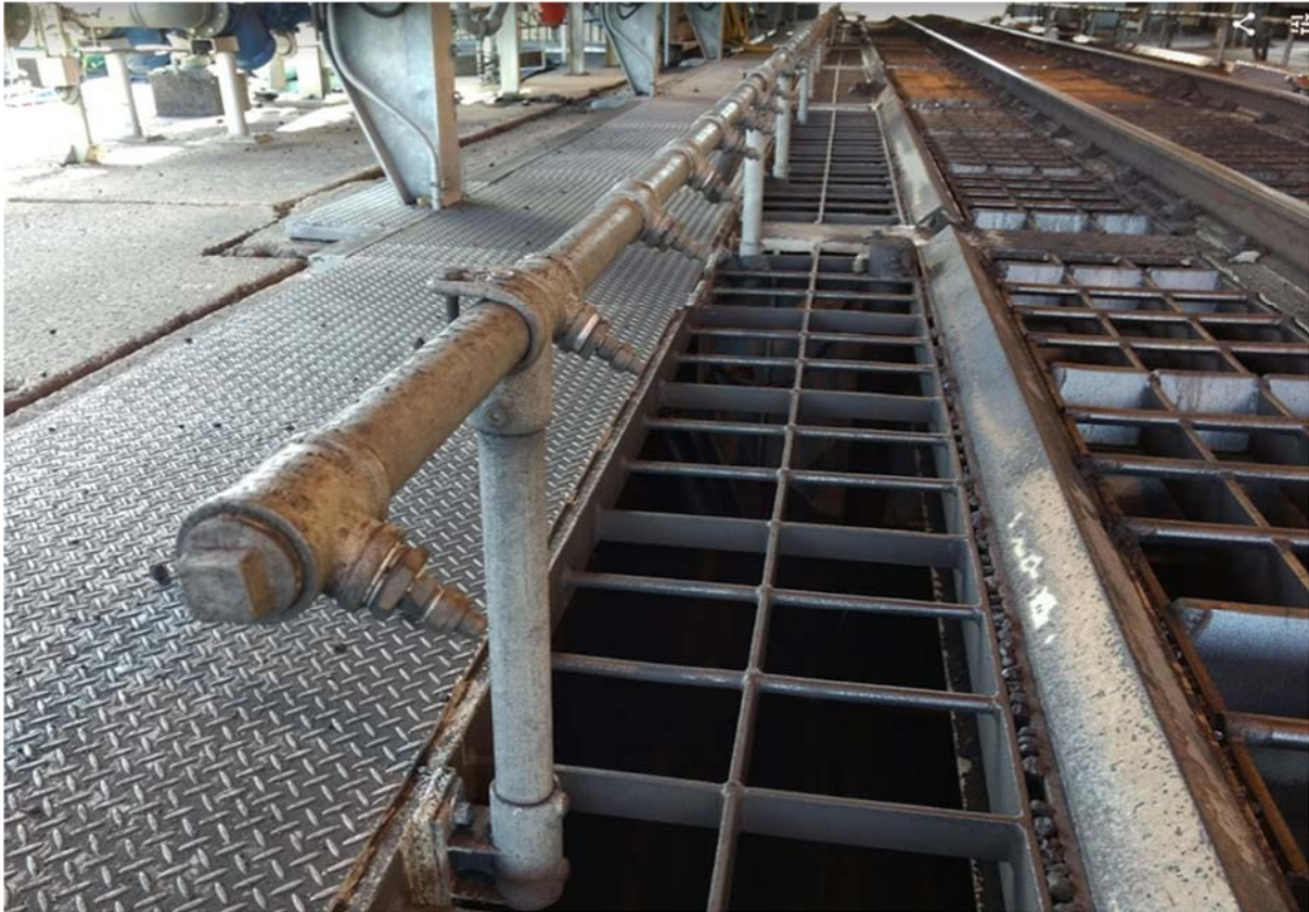
Image 1. Primary dust suppression at coal unloading facility.
