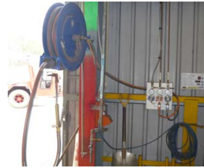
Reticulated gas/oxy supply to the workshop
