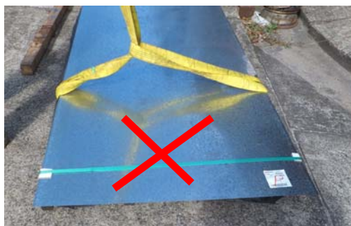
Figure 7: Unsafe use! Edges of metal sheet may cut sling
