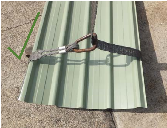
Figure 4: A steel webbing sling being used to lift roof sheeting – edges will not damage this type of sling
