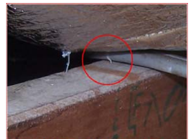
SHOCK HAZARD - Electrical cable pierced by a staple, energising the foil insulation
