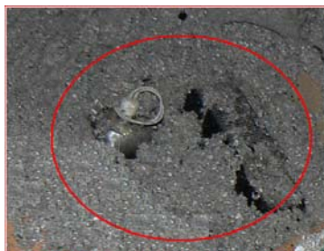
FIRE HAZARD - Halogen downlight and transformer covered with loose fill insulation
