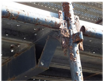
Figure 9 Severe corrosion on critical scaffolding components
